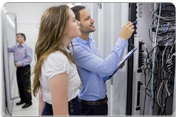
Installations must be inspected for damage.
